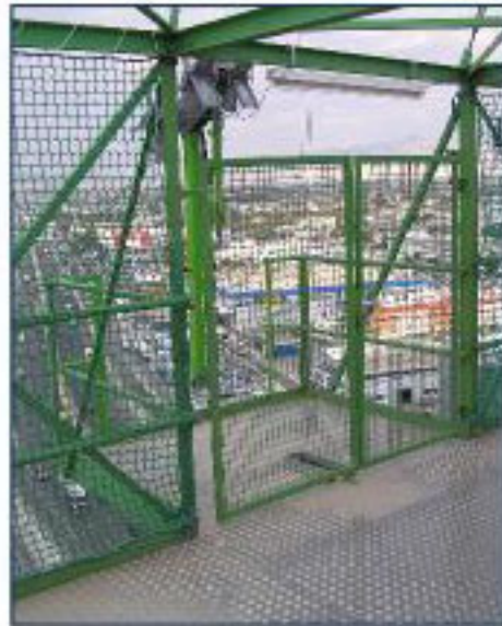
Launch ramp gate
